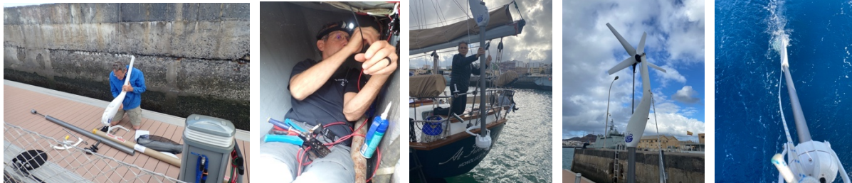
Boys and their toys. Installing the DuoGen® air and sea generator was surprisingly straightforward, and it did not require drilling any holes into the boat. It will give us the ability to keep our batteries fully charged overnight while on passages.
