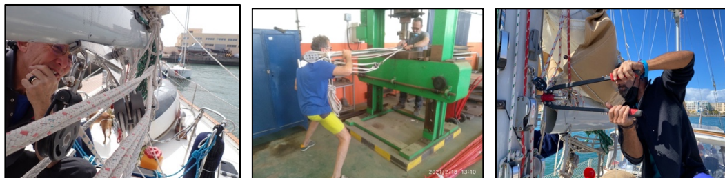
Repairing the gooseneck and vang was a mix of DIY and pro work. We needed a machine shop to straighten the bent tang on the vang, and riggers with extra-large Monel rivets to reattach the gooseneck.
